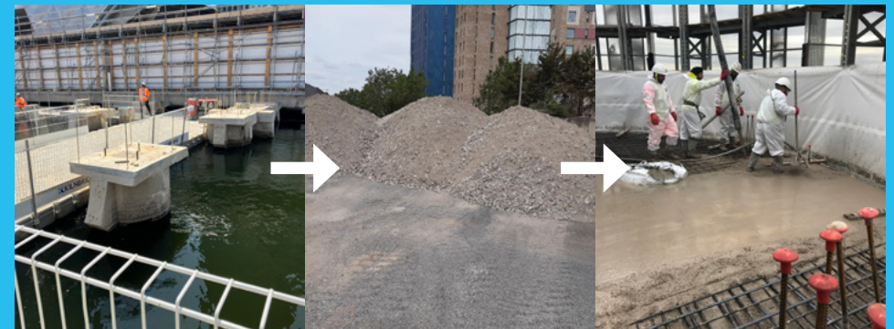
Concrete from North Quay identified, processed and re-used on site and at Wood Wharf
